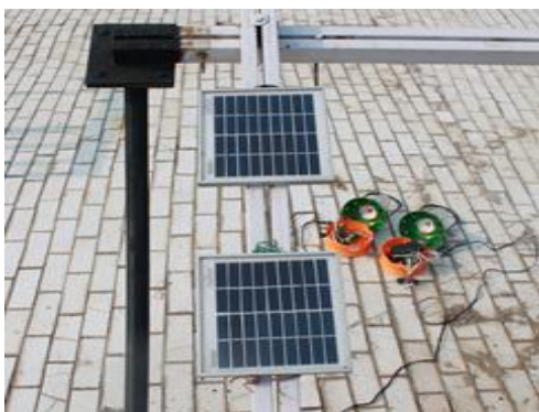
Figure 2: Battery charging station at SLL, TERI
