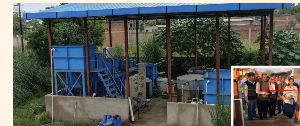
20 KLD tadox® WWT plant in Textile CETP, Kanpur under 'Namami Gange' Program; Inauguration by DG NMCG - Feb, 2023.
