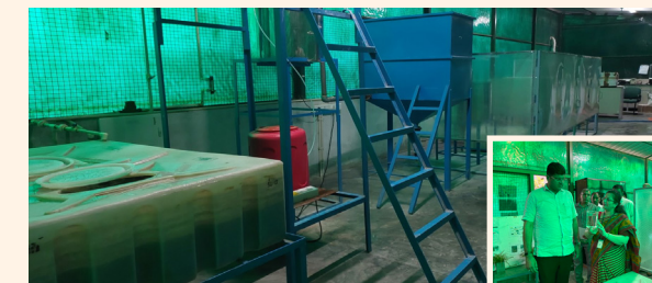
10 KLD tadox® WWT plant treating mixed sewage in TERI, Gurugram since Aug. 2020; Visit by Dy CM Haryana - October, 2022
