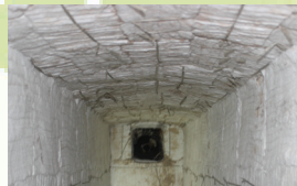
Furnace hot face insulation
