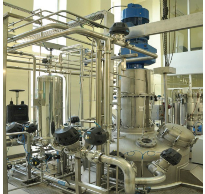
Oilzapper production plant at TERI Gram
