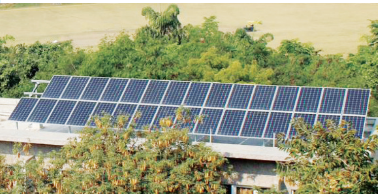
280 kWp solar rooftop installation at TERI Gram to meet the campus electricity needs
