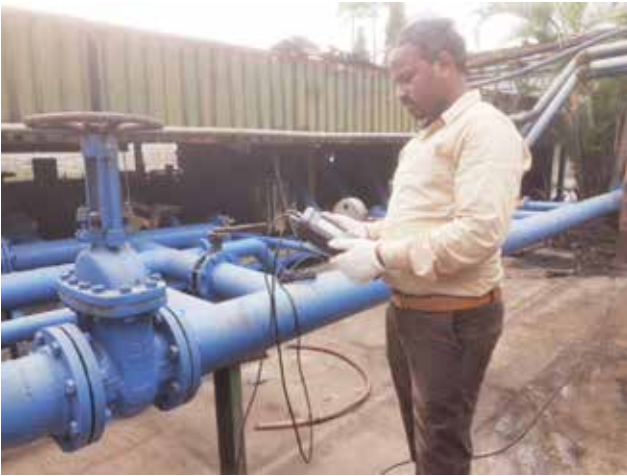
► Performance evaluation of cooling towers to ensure water and energy savings potential
