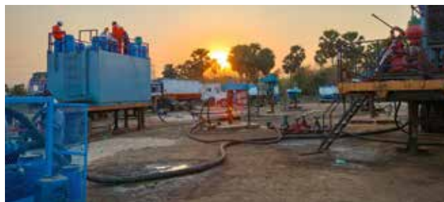
► In situ stimulation job for enhanced coalbed methane production at EOGEPL well site
