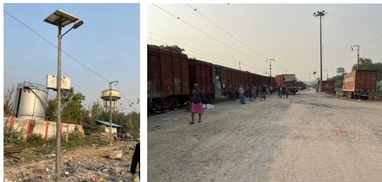
Lighting at Kishanganj
