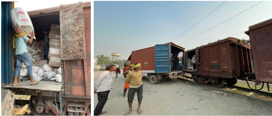
Loading/unloading area – truck to wagon
