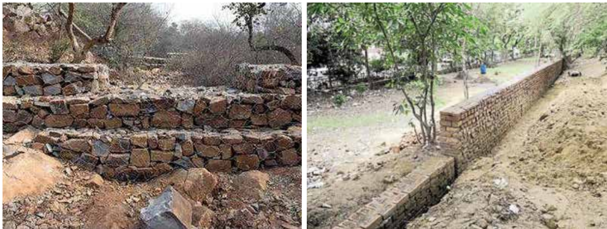
Figure 21 : Dilapidated traditional dams (bundhs) in Aravallis
