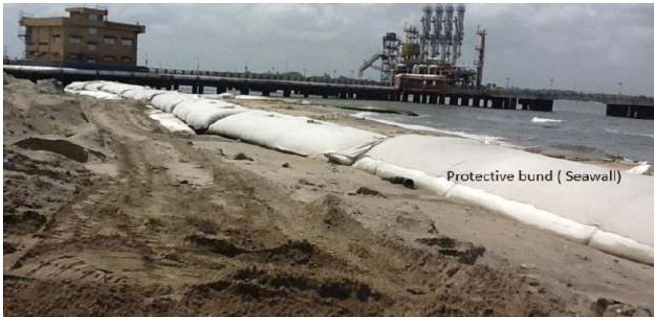
x. Construction of beach protection bund and groyne using geotextile tubes Kochi, Kerala, India
