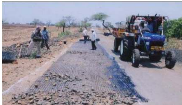
i. Laying of geo-grid for subgrade stabilization, Gharni-Nitur-Nilanga Road SH-167, Taluka-Nilanga, District-Latur, Maharashtra.
