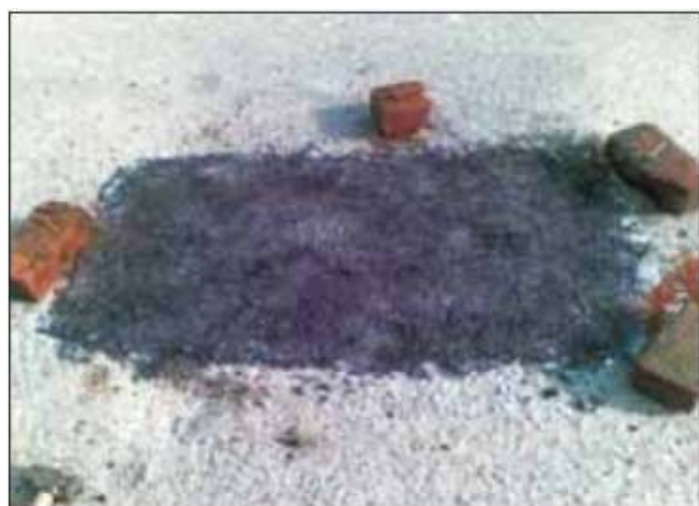
v. Pot hole, after its repair at Sukhdev Vihar road, New Delhi
