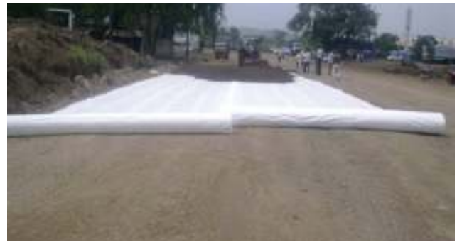
vii. Geotextile for separation, filtration and drainage (as per IRC: SP: 59-2002 & MORTH Clause-700) at Link Road between Paithan Road to Nagar Road (CH 0/000 to 4/041 including Bridge at CH 3/270 to 3/340) Taluka/District-Aurangabad, Maharashtra
