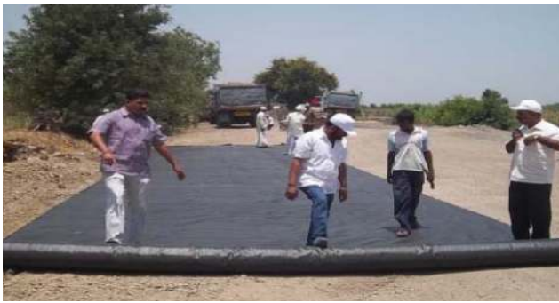
vi. Geotextiles in Road Construction and Prevention of Soil Erosion for Sub grade Stabilization at Jejuri - Morgon Road MDR-65, Taluka-Purandhar, District-Pune, Maharashtra
