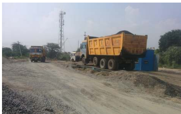
Photo 4: Weighing of bituminous mix for the periodic maintenance of the Orai–Barah section of NH-25
