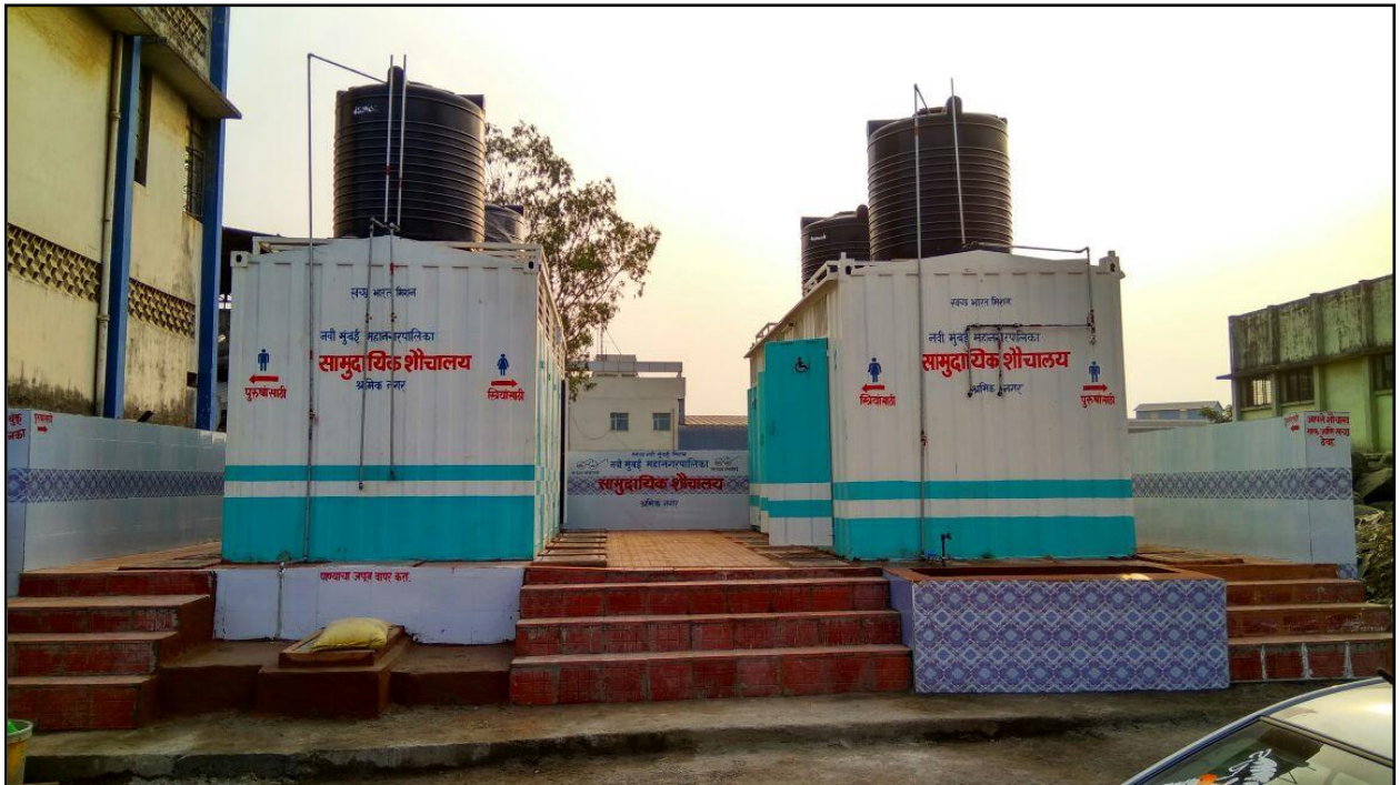
Picture No. 3: Community toilet facilities installed by NMMC
