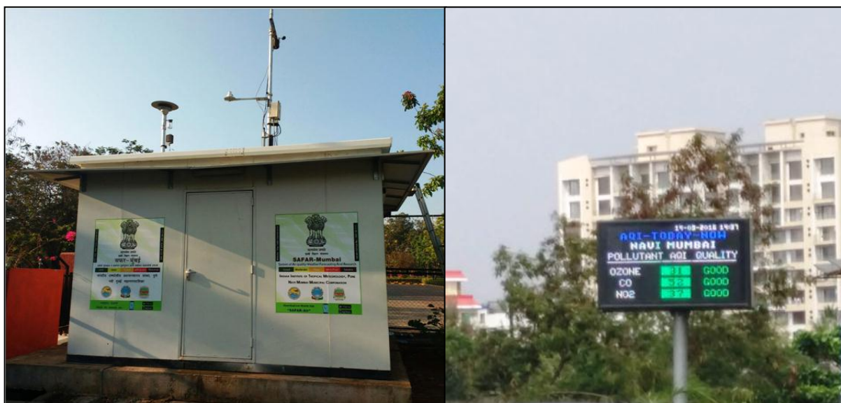
Picture No. 3: New CAAQMS installed at Wonders Park, Nerul
