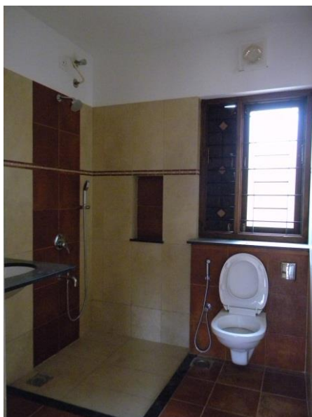
Figure4.13: Water efficient features depicting water closet and faucet
