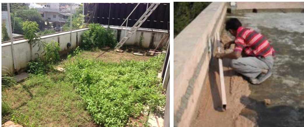
Figure7.11: Left: Terrace garden roof image Right: Insulated roof during construction (Image provided by Mr Kakani)
