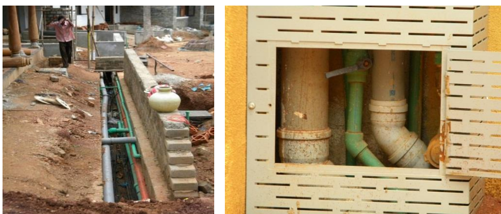
Figure4.4: Service corridor trench on site and plumbing service line in each housing unit
