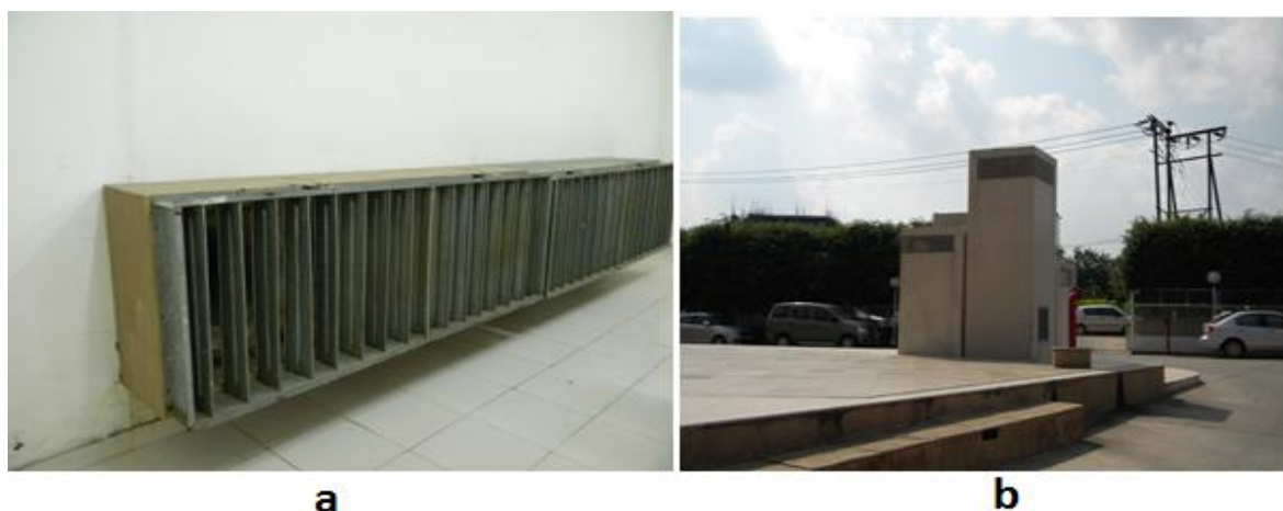
Figure8.22: a) Inlet to AHU from tunnel. b) Earth air tunnel intake chamber.
