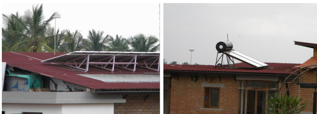
Figure 4.22: Solar Hot Water & Solar Photovoltaic panels integrated on roof top
