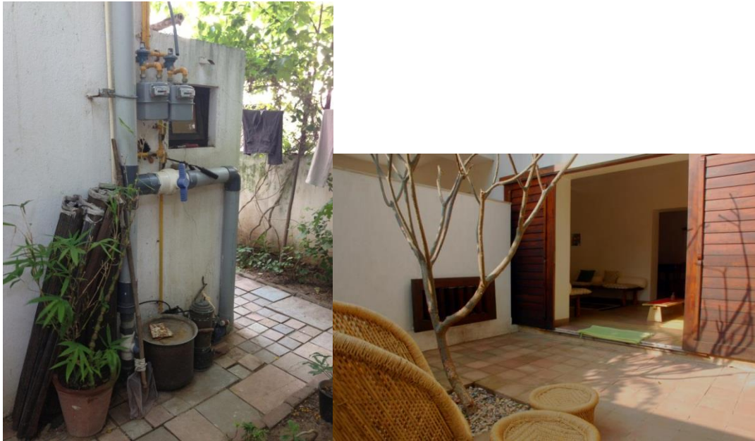
Figure7.23: Left: Rain water system plumbing lines, Right: Soft scape for rainwater recharge
