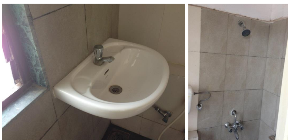
Figure 7.35: Water efficient features depicting water closet and faucet
