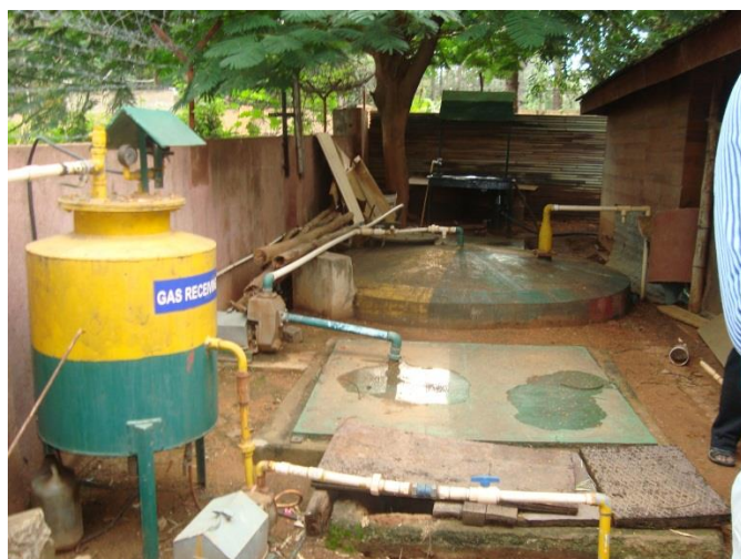
Figure 4.49: Bio digester plant
