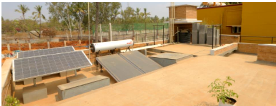
Figure4.39: Solar PV cells and Solar water heater
