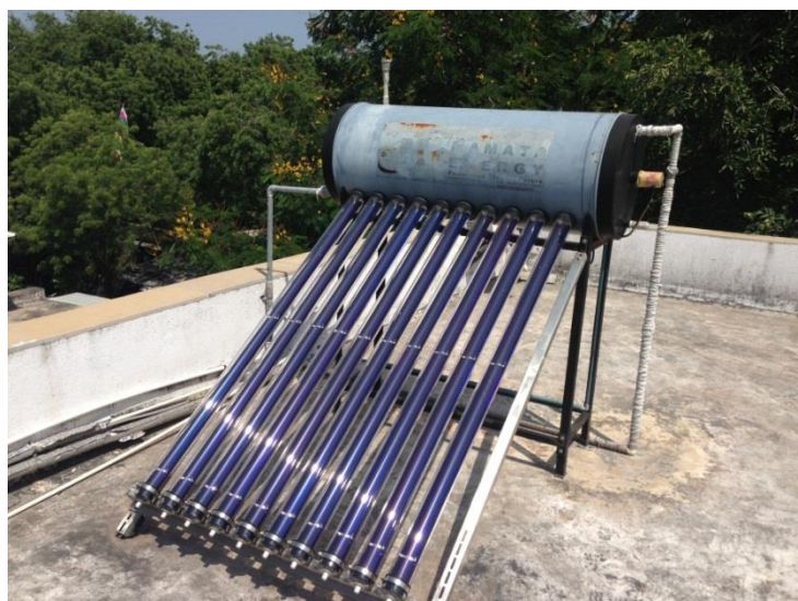
Figure7.21: Solar water heater on terrace
