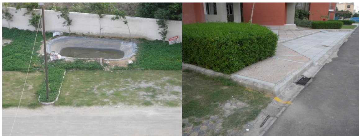
Figure 8.8 Sedimentation tank and storm water drain
