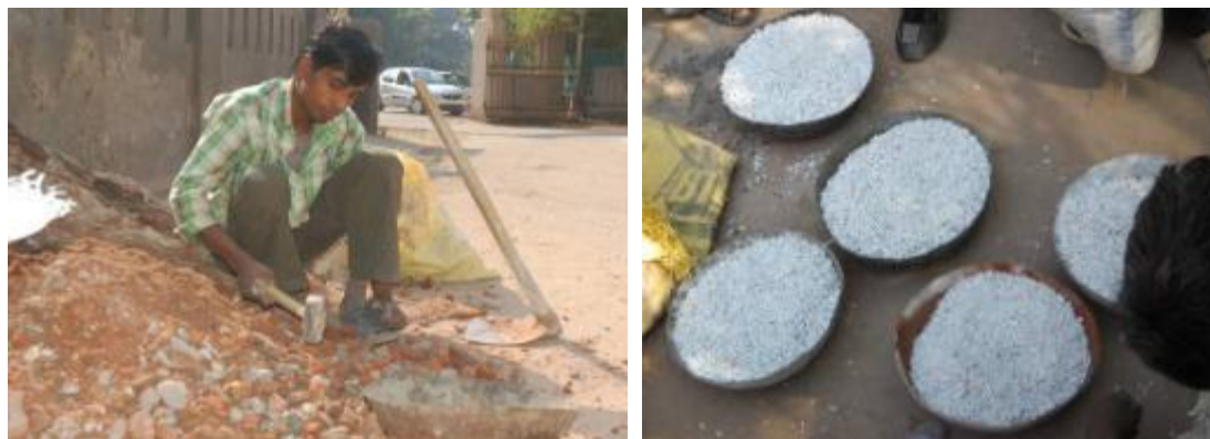
Figure7.12: left: demolished wall's construction waste used for roofing, right: thermocol waste for insulation (Images provided by Mr Kakani)
