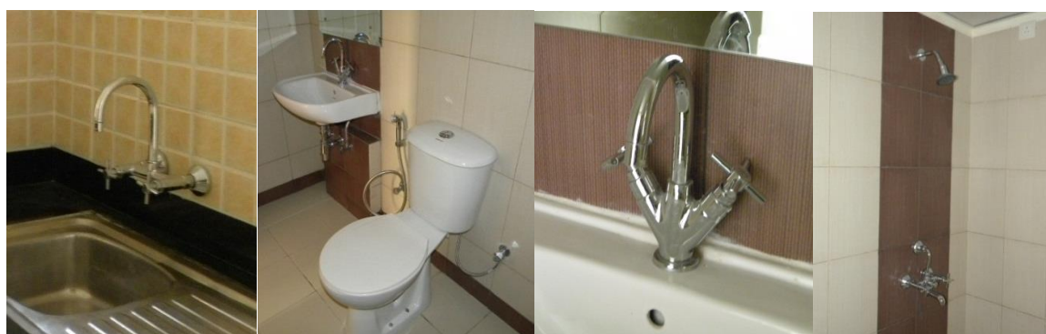
Figure 8.12: Images of various low flow water fixtures as seen during field visit
