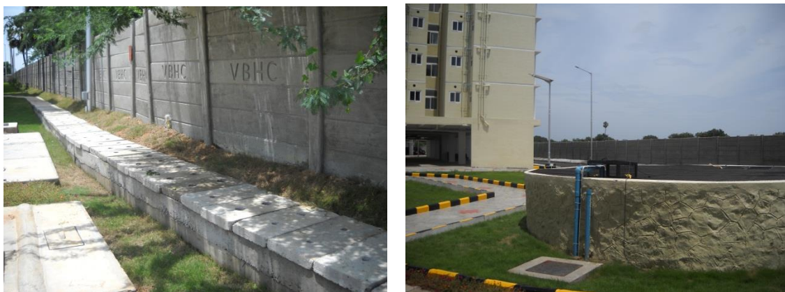
Figure5.9: Peripheral swales and the open well-constructed on site to collect the rain water.
