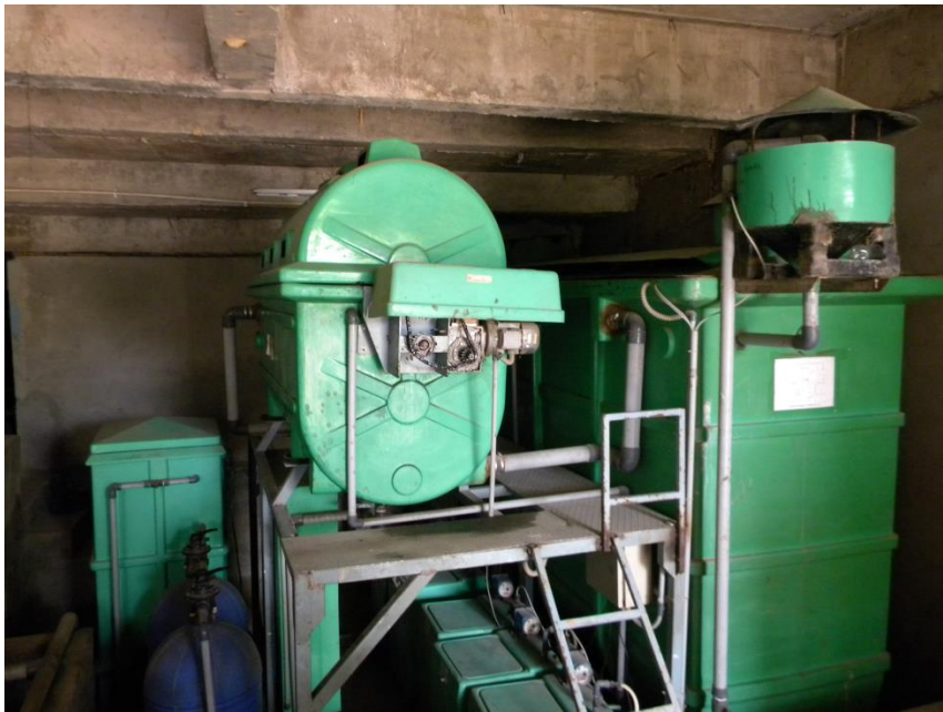
Figure8.18: a) sewage treats plant
