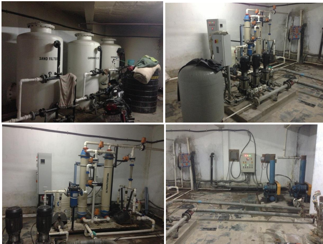
Figure 7.37: Photograph of Waste water treatment plant at Solaris
