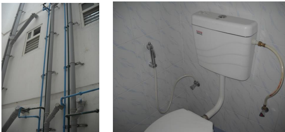
Figure5.10: Dual plumbing and dual flush toilets installed in the project
