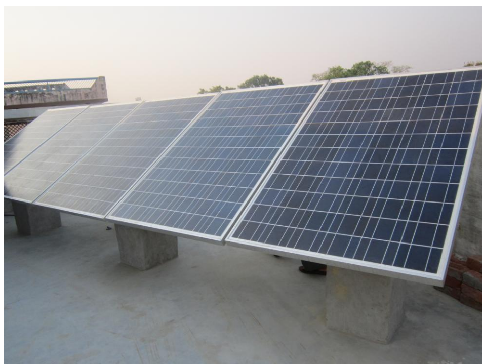
Figure 3.3 Solar photovoltaic panels
