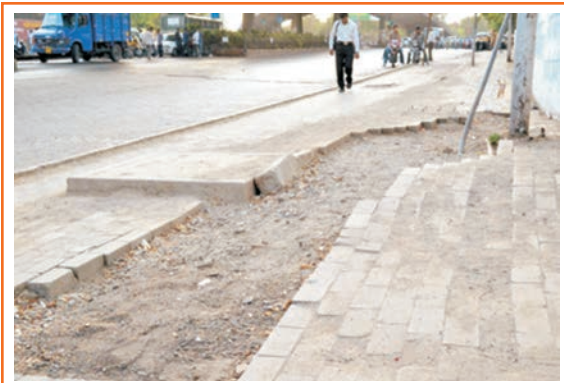
Photo 2: Poor maintenance of cycle track Source: http://www.mid-day.com/news/2012/jun/060612-Pune-News-Unusable-cycle-tracks-in-Pune-puncture-cyclists-enthusiasm.htm
