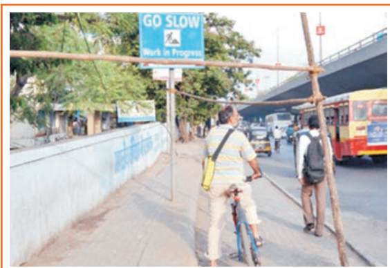
Photo 3: Obstruction on cycle track Source: http://www.mid-day.com/news/2012/jun/060612-Pune-News-Unusable-cycle-tracks-in-Pune-puncture-cyclists-enthusiasm.htm
